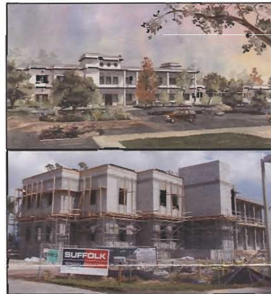
Under construction: Northern's new Administration Building and Emergency Operations Center is scheduled to be completed in September 2006.
