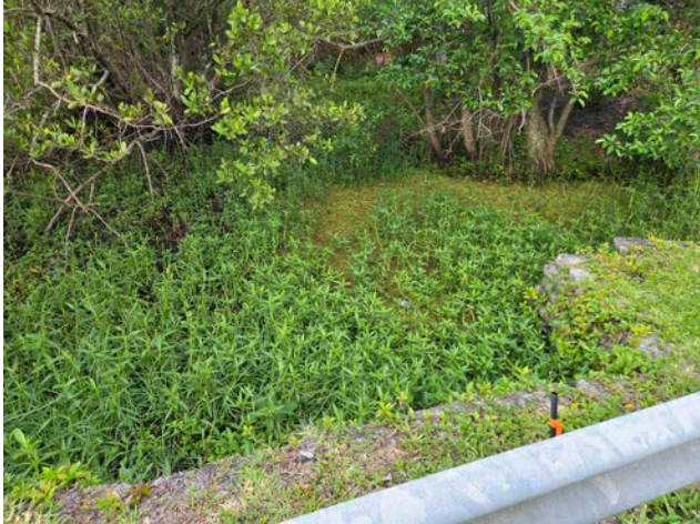
South side of Eagles Nest Drive — aquatic vegetation and duckweed backup at culvert outfall.
