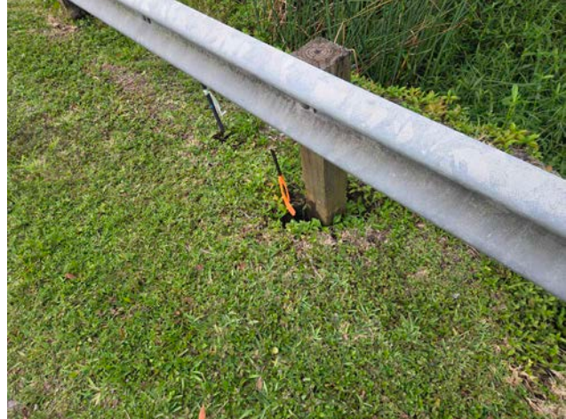
Ground subsidence adjacent to roadway safety barrier — evidence of underlying CMP collapse.
