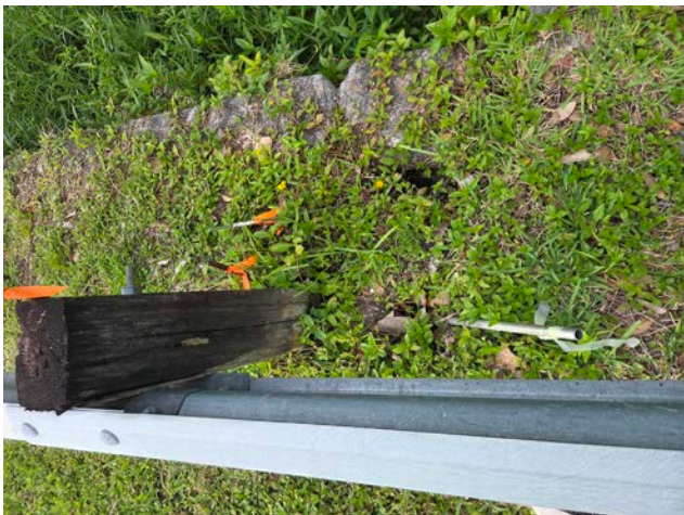
Close-up of void opening at guardrail post base — soil loss consistent with pipe failure below.
